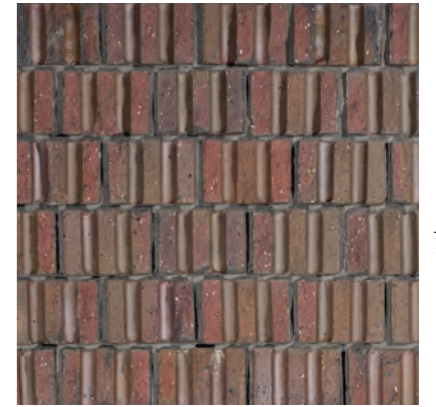
Breno FK6 broken with 2 gaps 120 x 85 mm
